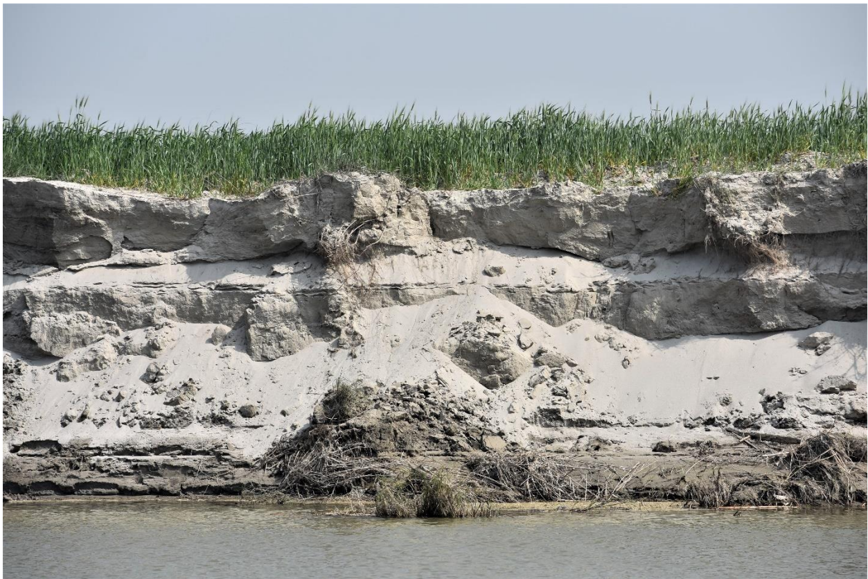
Image 23 : Ganga River Bank Erosion As Observed Near Kachhla Kham In Budaun Distt.
